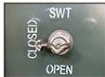
Load Break Switch
