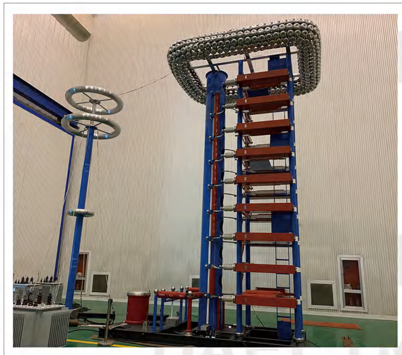
雷电冲击设备 Lighting Impulse Equipment
