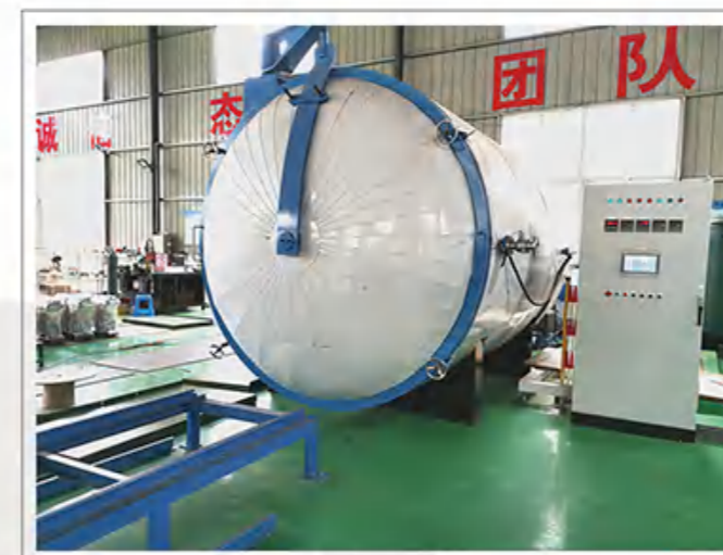
干燥箱 Transformer Drying Oven
